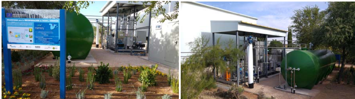
Figure 4: AnMBR demo plant constructed and installed
